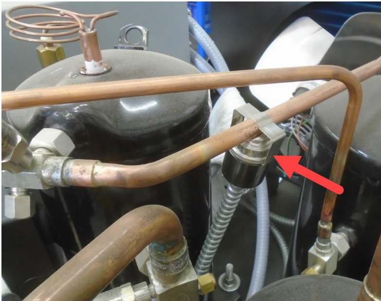
Figure 9: Discharge line thermostat.
