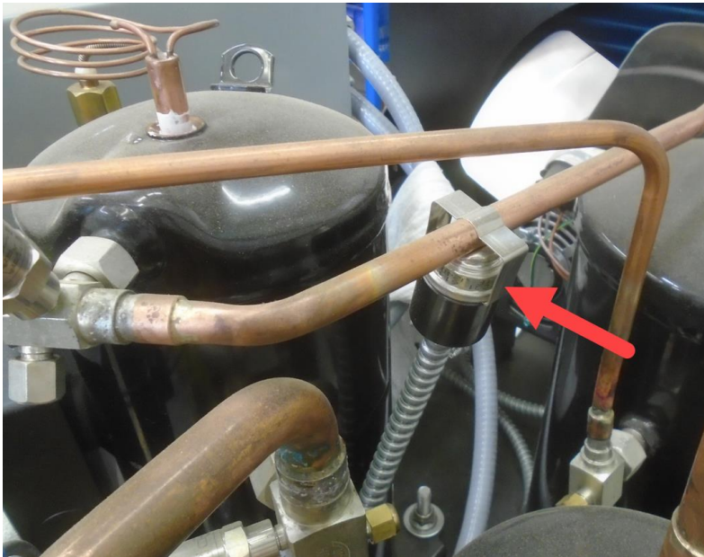
Figure 7: Discharge line thermostat.
